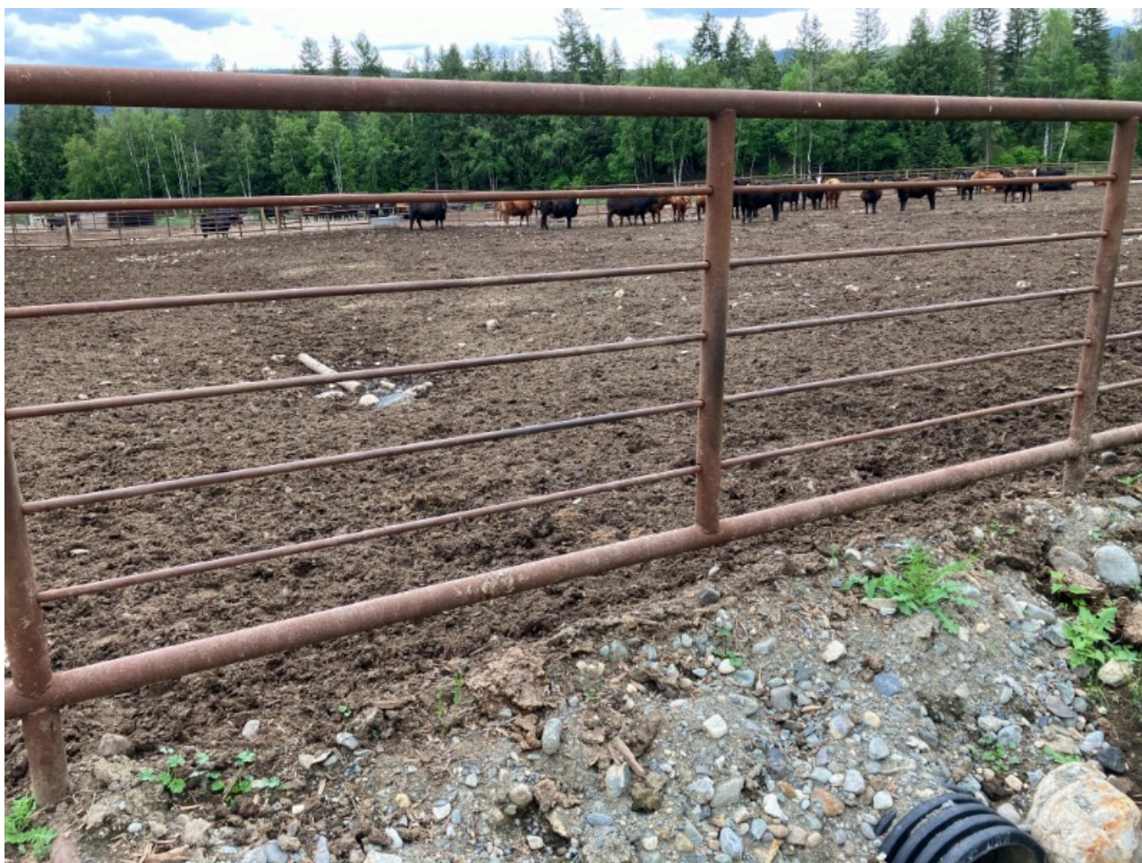
Photo 3. Drainage pipe within confined livestock area enabling contaminated runoff to escape.
